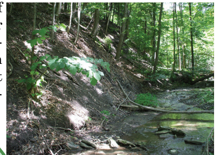
Tributary inputs from eroding streambanks such as from Rice Brook.
